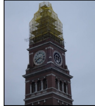
After many years of delays and false starts, restoration of Seattle's 1906 King St. Station is finally under way in earnest. Scaffolding
